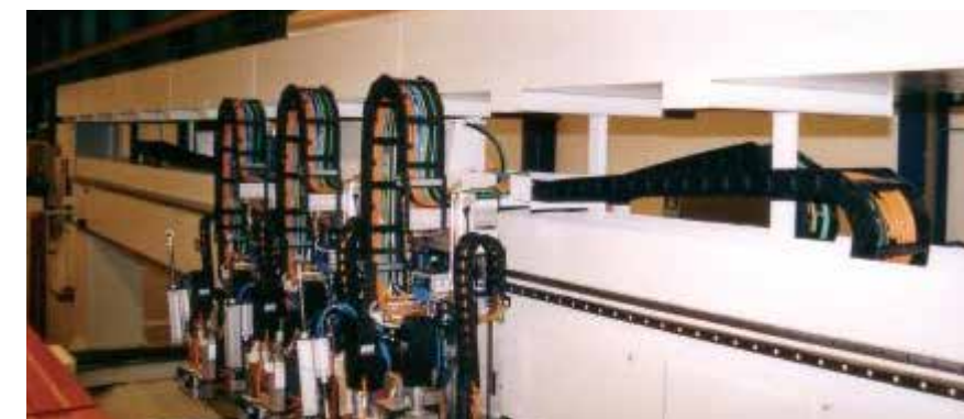
Woodworking machines with e-chains® and chainflex® cables
